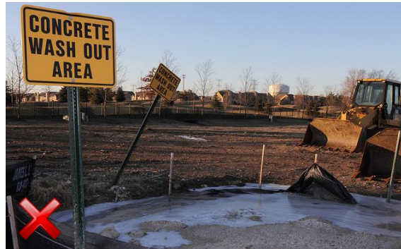
Poor job of containing washout inside of the designed area. Washout material should be removed when capacity becomes an issue.
