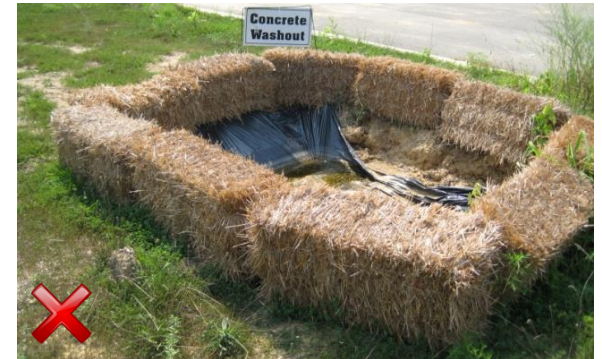
The polyethylene lining should wrap over the straw bales and be properly secured along the top. The lining used at this washout area is not thick enough.
