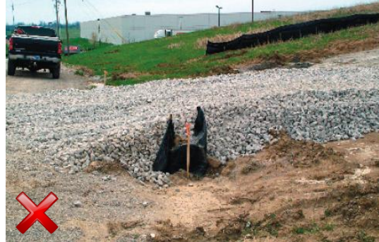
Drainage is maintained through the construction entrance by installing a temporary culvert beneath the gravel entrance. The area upstream of the pipe appears to have been stabilized, but the pipe outlet needs scour protection. Also, the lack of radius on the drive will prevent medium and large vehicles from entering and leaving the site.
