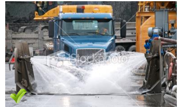
Larger sites that are hauling significant amounts of material to/from the site are better managed through more significant vehicle washing measures.
