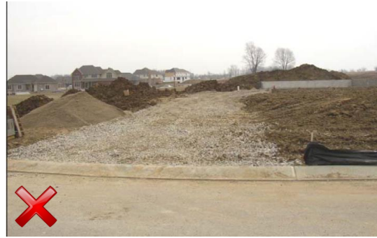
Example construction entrance at a small site. Notice the accumulation of sediment in the rock has resulted in transport onto the roadway. No diversion berm was installed to prevent sediment-laden runoff from flowing onto the roadway. Also note that the silt fence has not been properly turned uphill to prevent sediment washing onto the entrance and/or onto the public roadway.
