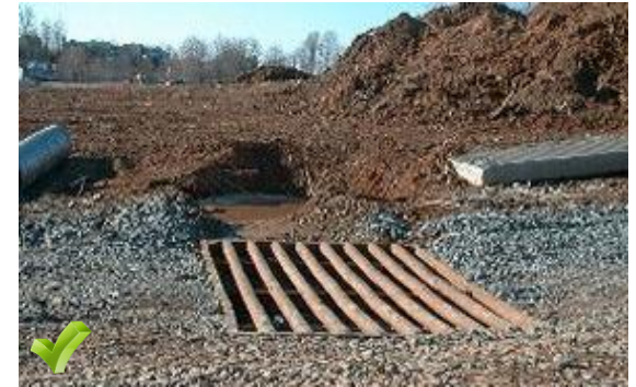
Example of a wet pit used for hosing of vehicles to minimize sediment deposits on the roadway. Note: The sediment collection traps must be periodically cleaned to remove accumulated sediment. Tire runoff must be diverted to an area on the site where it is detailed. These traps are only intended to collect sediment; they are not for excessively oily or greasy equipment.
