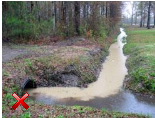
Improper discharge can be identified by foam or suds in the storm system.
