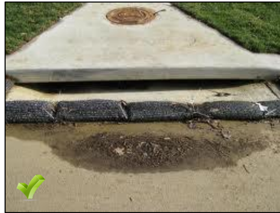
Provide inlet protection at curb inlets and/or catch basins around the building site. Never dispose of or deposit any substance into the storm collection system.
