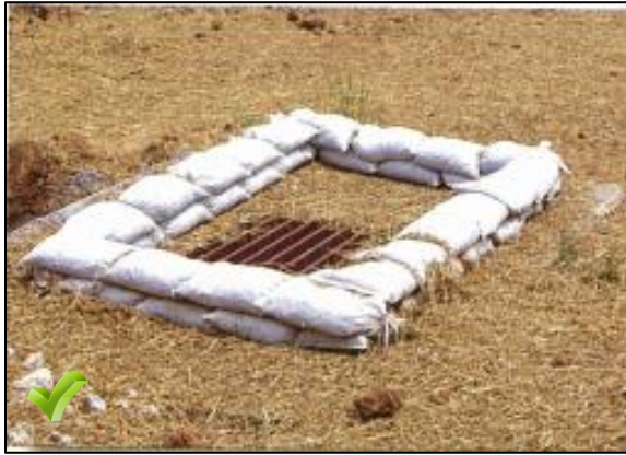
Inlet protection berm construction of half-filled stone bags. Use #57 rock, and overlap bags to eliminate large openings and rapid flow-through.
