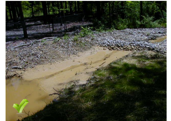
Good application of sediment trap installation. The stone spillway provides a stable overflow structure. Sediment basin is at capacity and should be cleaned prior to next storm event.
