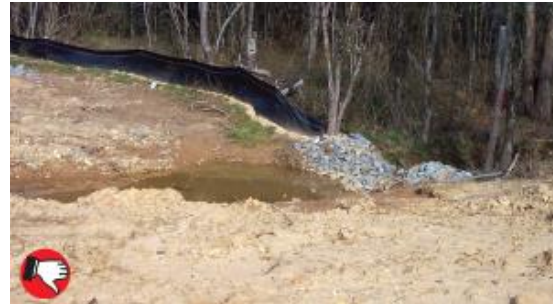
Example of poor trap installation. Overflow notch is too deep and surrounding area needs seed and mulch to prevent erosion.
