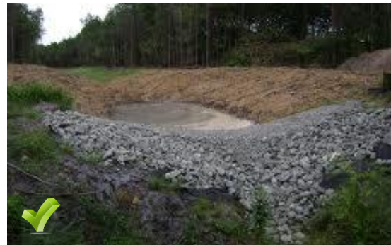
Good example of a sediment trap. Rock overflow notch is properly installed, and bare soil has been covered with seed and mulch.
