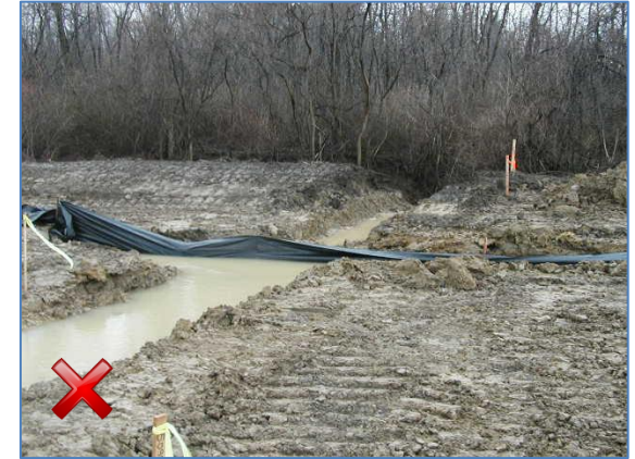
Example of poor sediment trap installation. Silt fencing should never be used as an outlet structure for a sediment trap.
