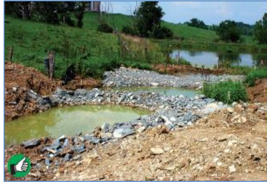
Fair installation of two traps above a small pond. Dikes are a little too small and the area needs seed and mulch.
