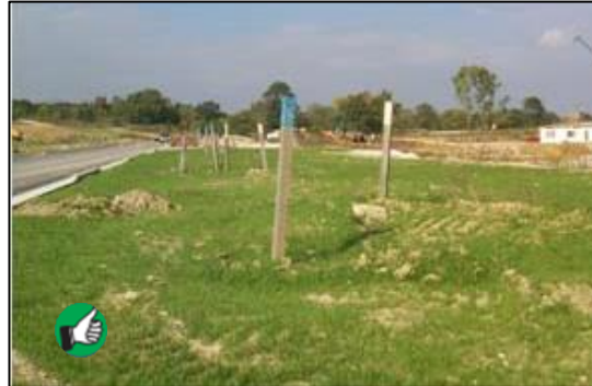
Example of temporary seeding to cover open areas where construction is not taking place.
