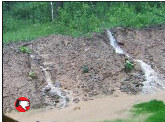
Temporary seed and mulch not applied to the slope. Erosion of soil occurs during rain event.
